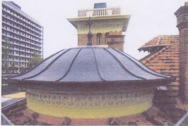
Repairs to the Old Observatory's oriel roof have been completed. G Pickering
